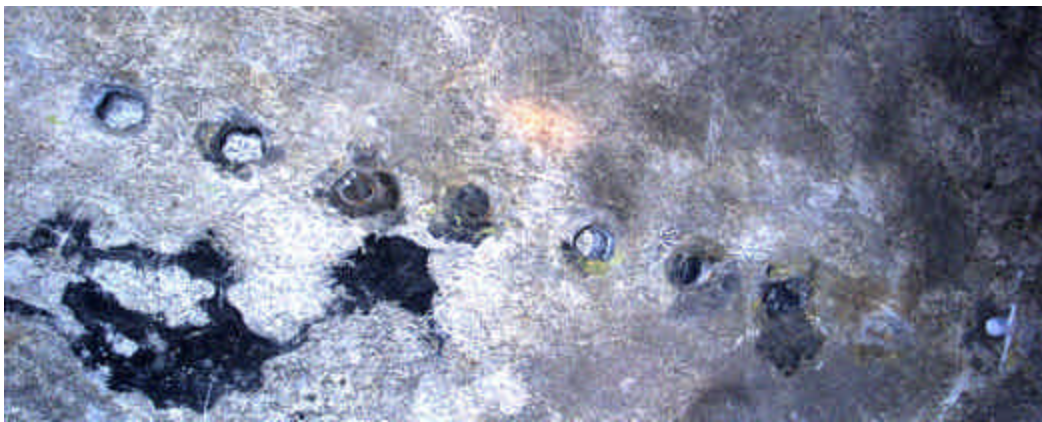
Figure 3. Holes drilled into the ceiling of Mammoth's Historic Entrance to accommodate bars of a previous gate.
